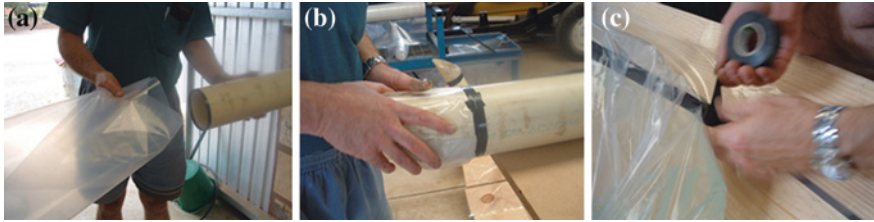
Fig. 11 Steps in making a poly plug-flow digester. a Folded layflat tube. b Inlet completed. c Fitting gas outlet tube
