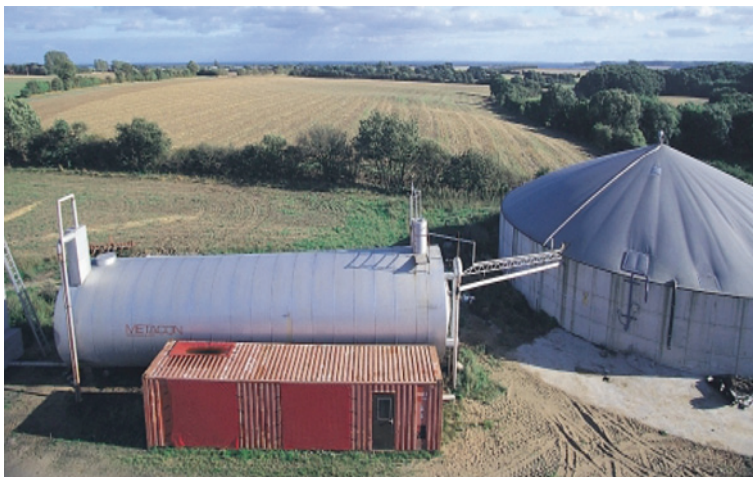
Fig. 3 Torsø farm biogas plant. “Blacksmith plant” with horizontal steel reactor (Photo by Landbrugets Rådgivnings-center, [48])
