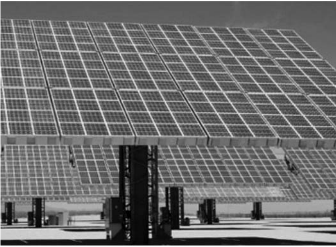
Figure 5.16 5 MW CPV System installed by Amonix trackers (Source: Amonix, Inc, reproduced with permission)
