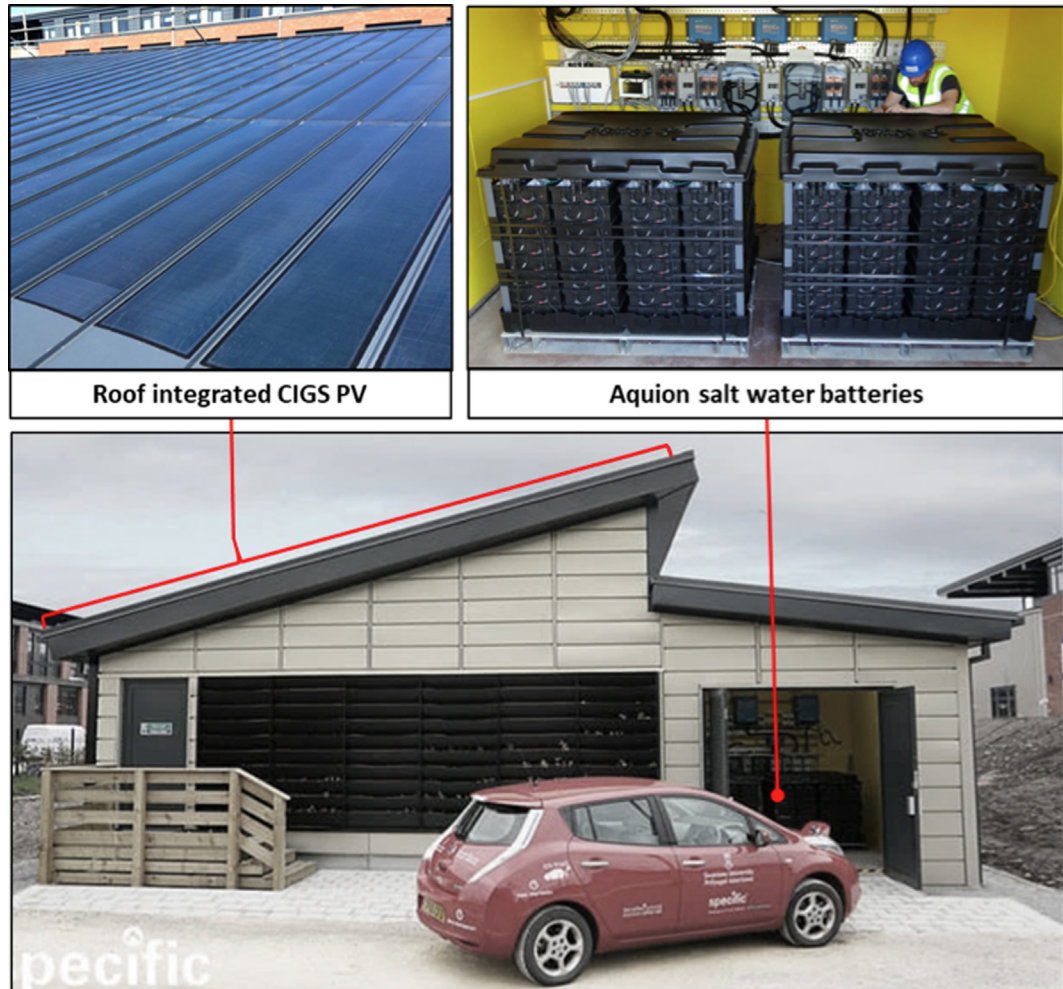
FIGURE 5.1 The SPECIFIC 'Active Classroom' with roof integrated PV and salt water batteries.
