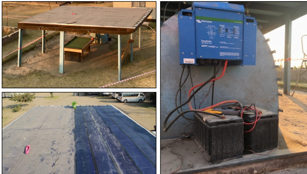
FIGURE 5.9 Photographs of the build in Mutende, Lulamba, Zambia 12 months after installation, demonstrating the problem dust can cause on PV systems in challenging climates. Dust accumulation on PV modules (left) and batteries and inverters, even in enclosed spaces (right), is a major problem.
