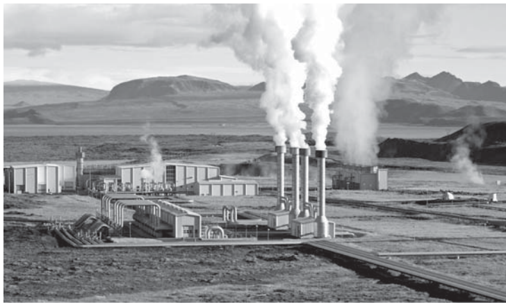
Figure 1.21 Nesjavellir geothermal power station, Iceland. Due the high concentration of volcanoes, Iceland has an unusual advantage of utilizing geothermal energy. Shown here is Nesjavellir Geothermal Power Station with a capacity of 120 MW.
