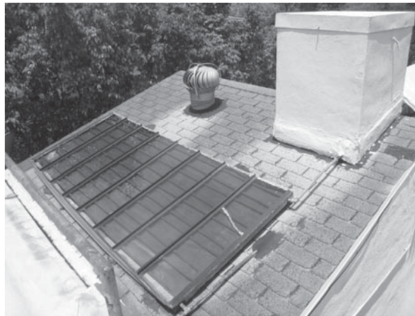
Figure 1.28 A Day-and-Night solar water heater in Florida. From 1920 to 1941, more than 25,000 solar water heaters were manufactured and installed in Florida. After 80 years, thousands of them are still working. The photo, taken by the author in Miami in August 2010, is a solar water heater installed in 1937. The insulated water tank is disguised as a chimney. Even with a broken pane, it is still working properly.
