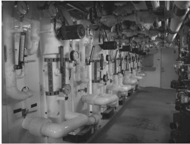
Figure 6.12 Heat pumps in the basement of Knox Hall. A photo taken by the author in the basement of Knox Hall, Columbia University. An array of heat pumps are shown on the left-hand side. The right-hand side is ground-well connections. Deep in the ground, the temperature is always at 57°F (14°C). In the winter, the heat pumps extract heat from the ground to warm the rooms. In the summer, the heat pumps extract heat from the rooms and dump it into the ground. The investment can be recovered in about 7 years from saving electricity. Courtesy of Columbia University.
