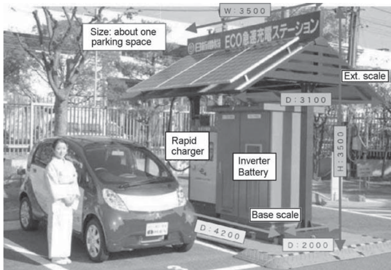
Figure 12.10 Solar-powered electric car charging station in Kyoto. The charging station, supplied by Nissin Electric Co., has a battery pack, an inverter, and a rapid charging setup. Courtesy of Kyoto University.
